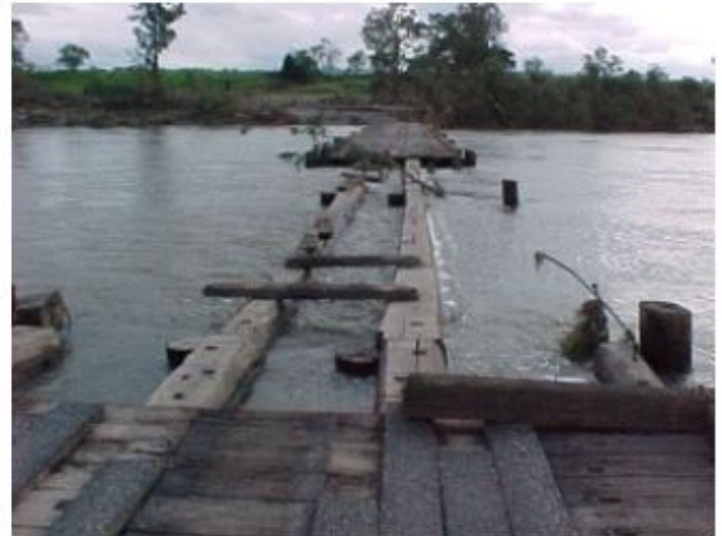
Tuimers Flat Bridge damage detail
