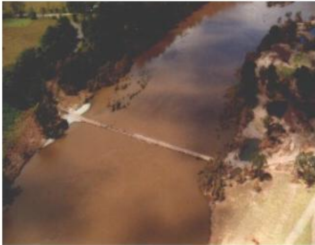
Tuimers Flat Bridge - Span missing
